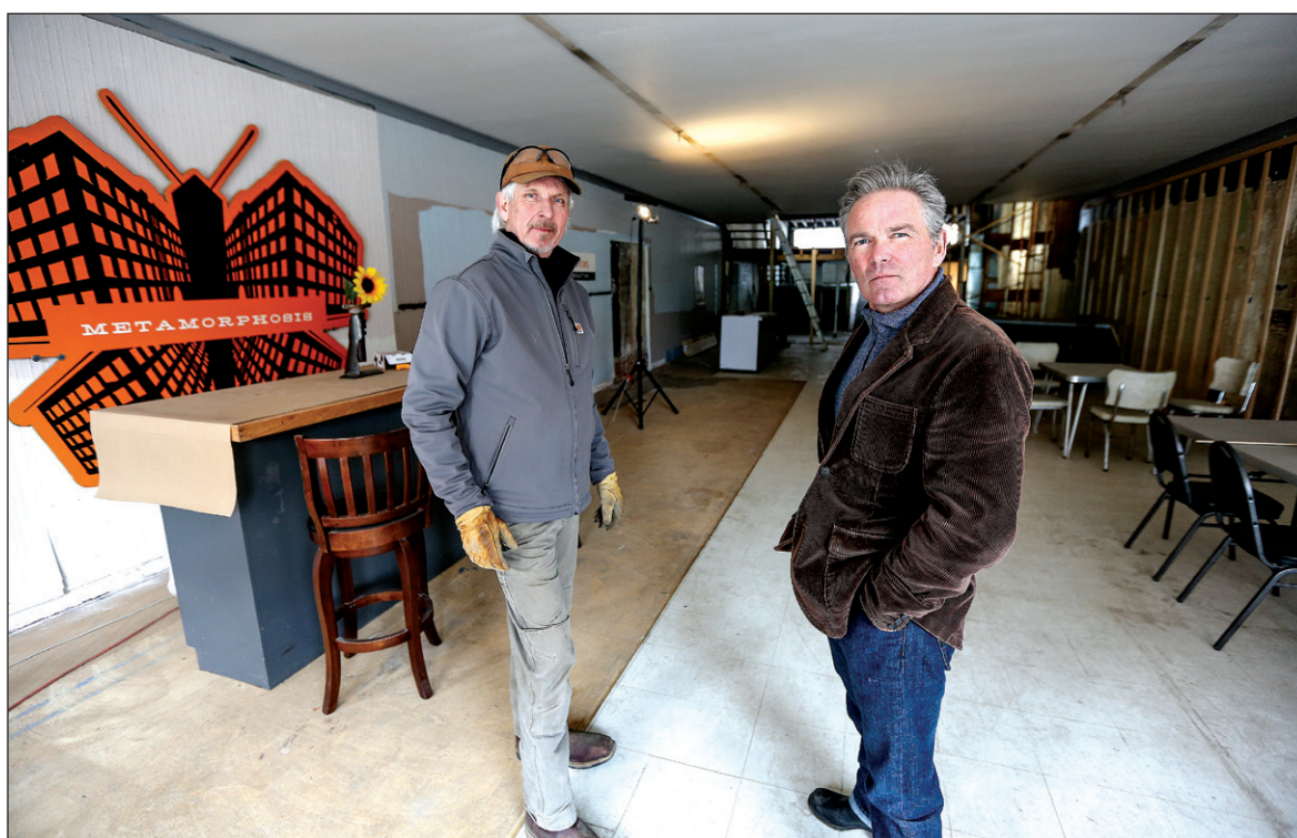
Gene Tully and Sam Mulgrew are working on the construction of the new location of Voices Studios on
