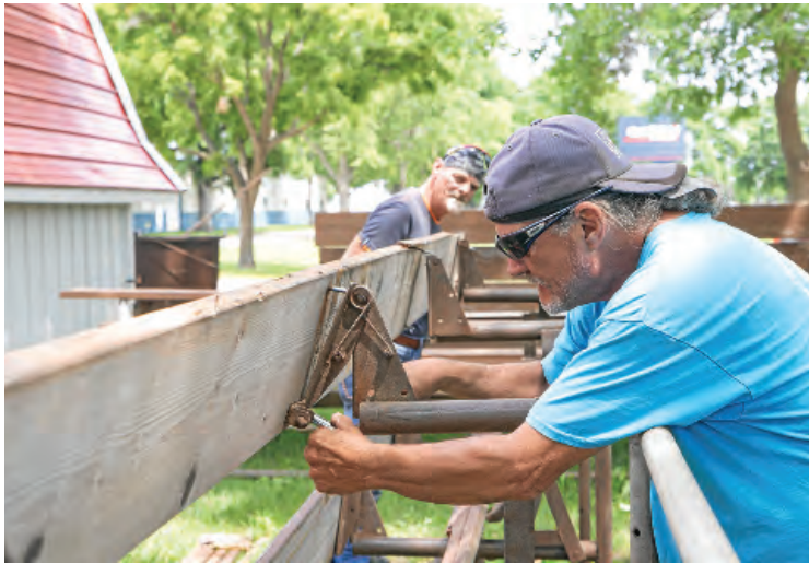
Randy Johnson removes the old bolts on these bleachers to install new boards as they prepare for the Clay County Fair in Spencer, Iowa.
