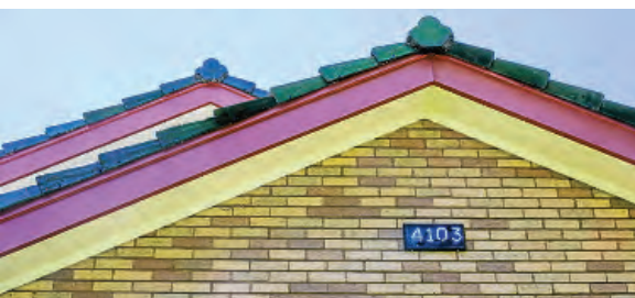
Restored neon house numbers are shown at the Tom and Cyndi Tener residence.
