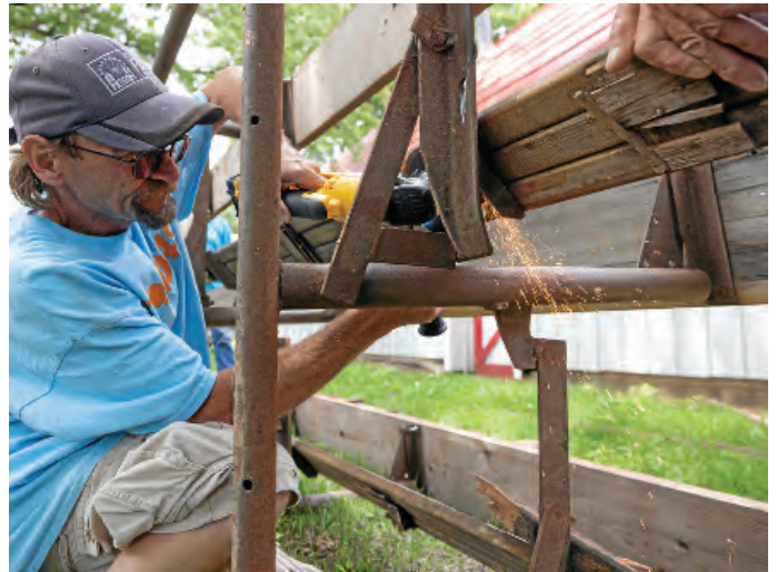
Dan Alspach cuts off rusty bolts in order to install new boards and modernize these bleachers before the Clay County Fair opens.
