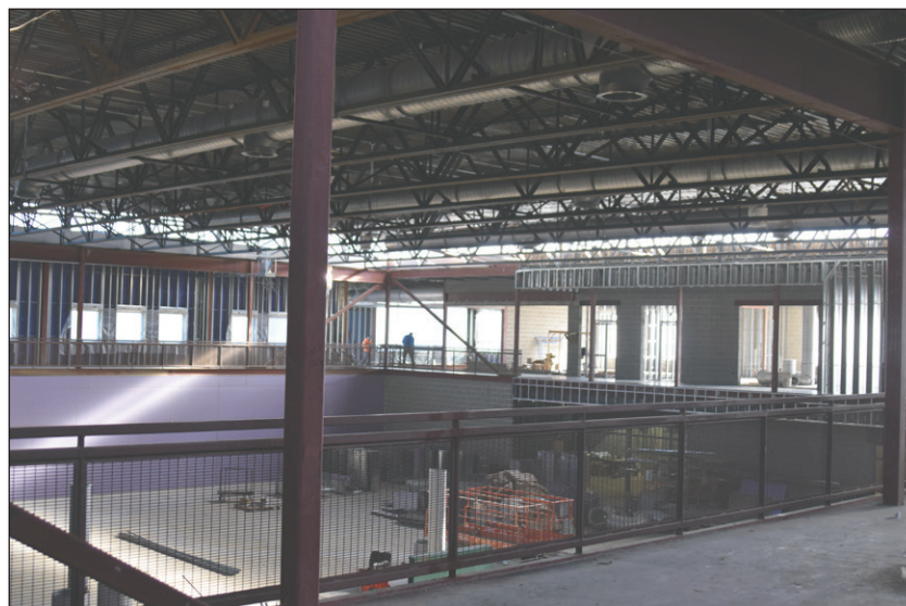
Jamee A. Pierson/Jasper County Tribune With space for two full basketball courts, the new gym will be another jewel for the school following the addition of the new football stadium last fall.
