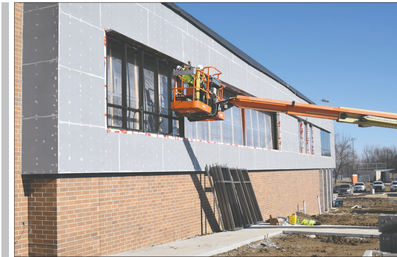
Crews work on the exterior of the new addition to Colfax-Mingo High School.
