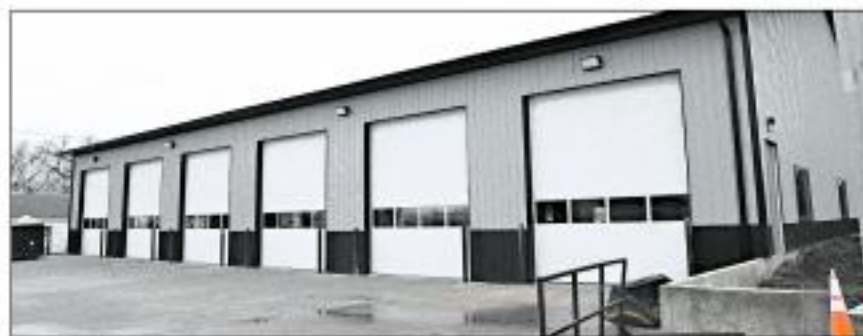
A new building is under construction to house the Boyden Fire & Ambulance by early 2023. The other half will be used as a bus barn for the Boyden-Hull School District. An anonymous group is putting forth money for the project. Photo by Eric Sandbulte
