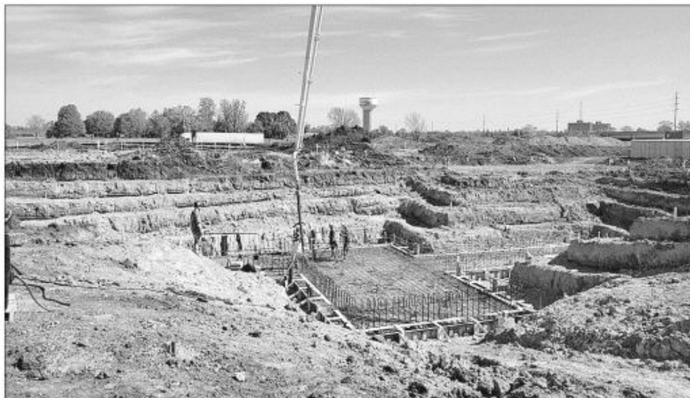
The Iowa State University Kent Corporation Feed Mill and Grain Science Complex is being constructed on 10 acres of land in southwest Ames. The Iowa Board of Regents approved a $24 million budget, but the final figure may be closer to $30 million. Photo submitted
