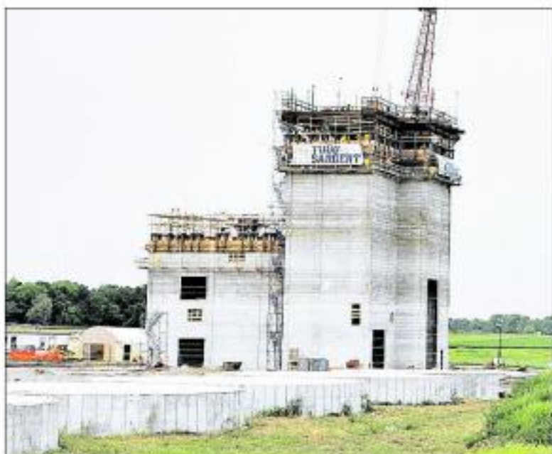
Work continues on a multimillion dollar, full-size feed mill and research facility at Iowa State University south of Ames. The ISU Kent Corporation Feed Mill and Grain Science Complex is scheduled to open in 2023. Photo submitted
