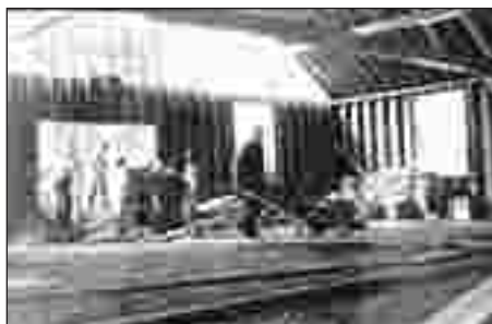
Contributed by Lucille "Susie" Leppla Wilhelm Family, friends and neighbors help pour the concrete floor.
