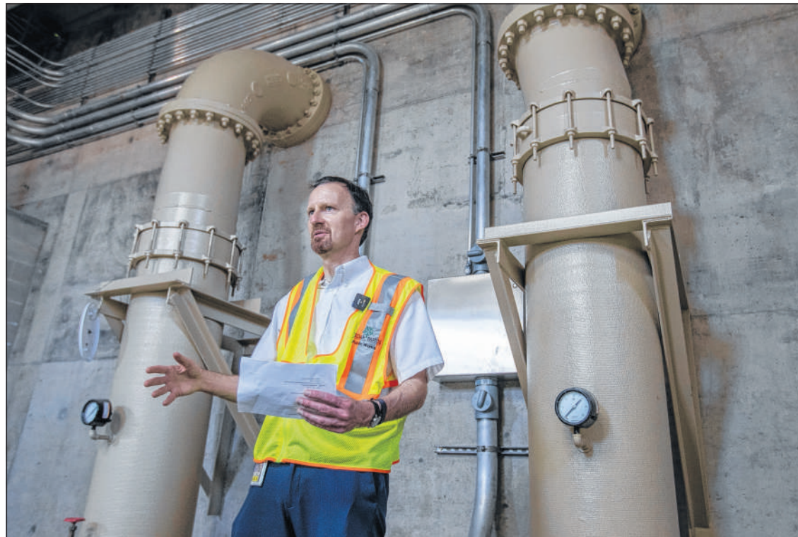
Cedar Rapids Flood Control System Manager Rob Davis talks May 23 about the uses of the pipes behind him at a pump station in NewBo in Cedar Rapids. (Savannah Blake/The Gazette)
