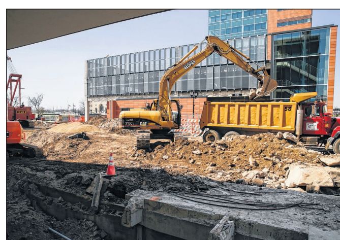
Work is underway on the Third Avenue SE floodgate on April 5, 2021, in Cedar Rapids. The floodgate features stackable panels that can take up to eight hours to erect. (Jim Slosiarek/The Gazette)
