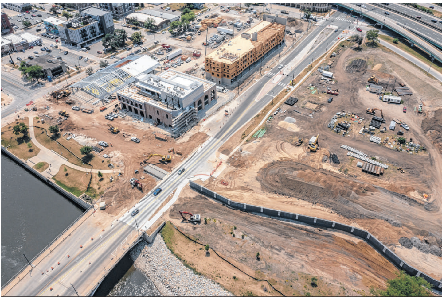
Construction work continues Thursday on a flood wall and a mixed-use development along First Avenue W in Cedar Rapids. The city accelerated work on a flood wall, seen in the bottom right portion of this aerial photo, between First Avenue W and E Avenue NW to align with construction of the Pickle Palace bar and grill and Big Grove Brewery on the nearby mix-use First and First West development. (Nick Rohlman/The Gazette)
