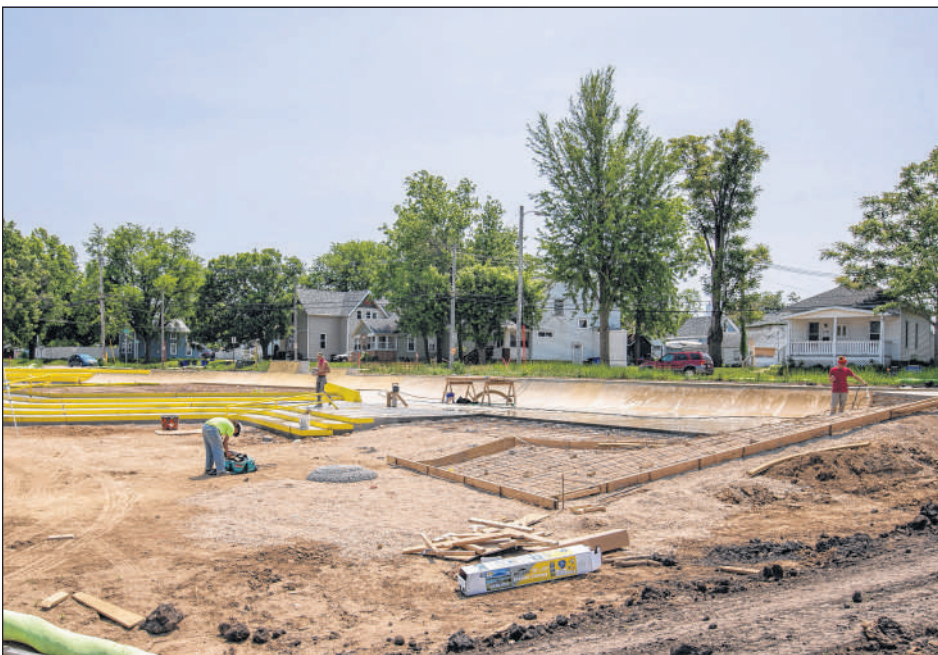
Crews work May 23 on the new skate park at Riverside Park in southwest Cedar Rapids. The city is constructing a detention basin where the playground and skate park once stood, so the city is moving the skate park and park close by. (Savannah Blake/The Gazette)
