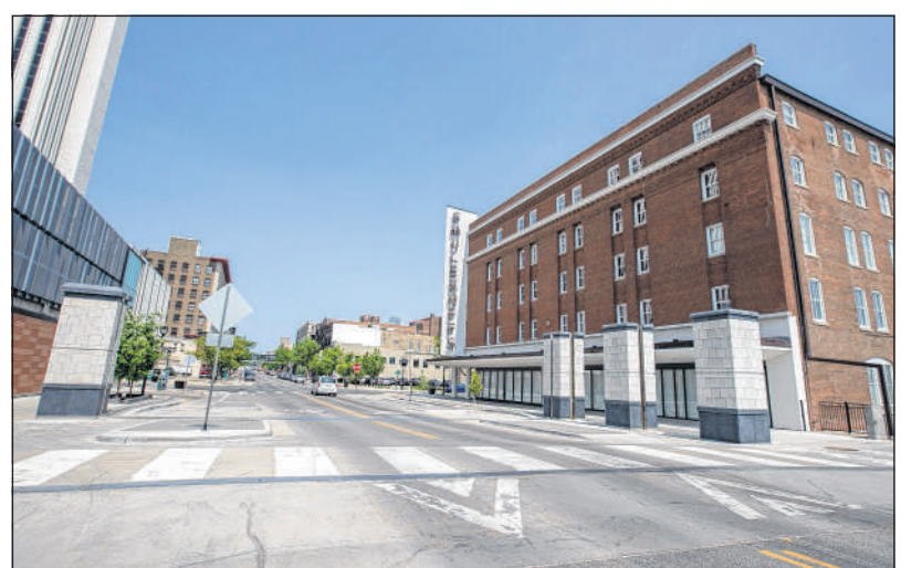
Posts for removable flood walls and gates are shown in May along Third Avenue SE in Cedar Rapids. (Savannah Blake/The Gazette)
