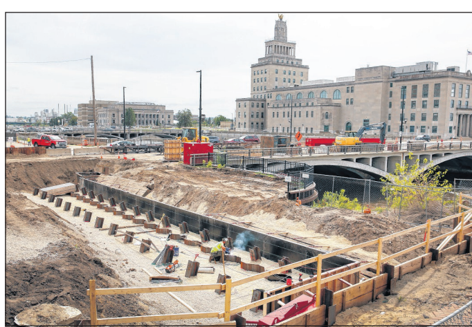
A worker welds tie backs for concrete forms into place as construction continues in September 2021 on the foundation of a flood wall near the intersection of First Avenue NE and First Street NE in Cedar Rapids. (Jim Slosiarek/The Gazette)
