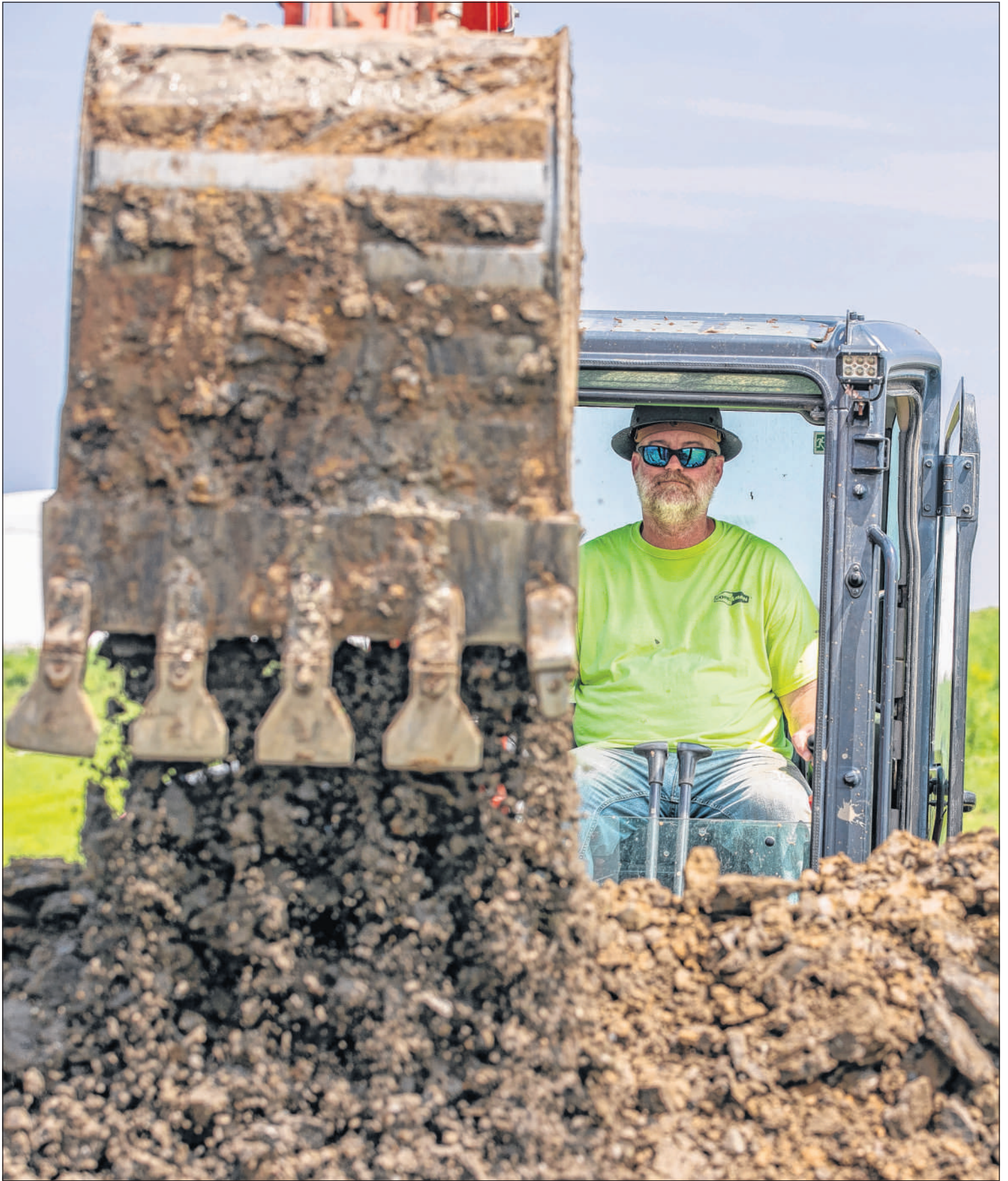
AONE Geothermal employee Justin Corkrean watches Wednesday as he digs a hole for a pipe at the new Cedar Falls High School in Cedar Falls. More than 20 acres of reconstructed prairie will encircle the school, along with four bioretention cells. The combined projects will absorb and treat an estimated 5.4 million gallons of stormwater a year — enough to fill about eight Olympic-size swimming pools. The water that doesn't run into the Cedar River lessens the potential for flooding downstream in Cedar Rapids. (Savannah Blake/The Gazette)
