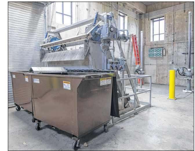
The inside of the pump station on Lot 44 in Cedar Rapids is seen May 23. (Savannah Blake/The Gazette)
