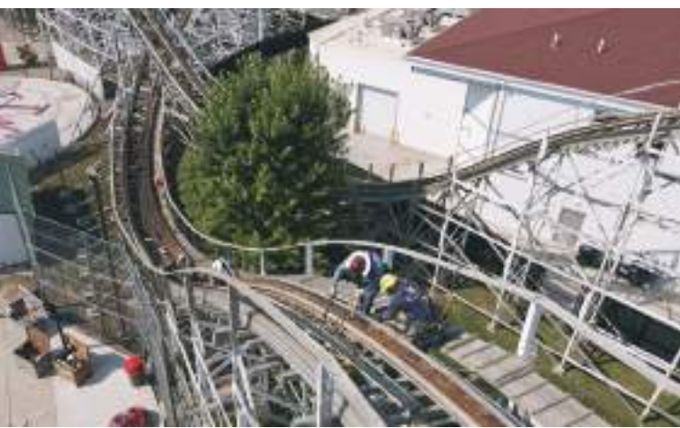
Crews began deconstructing portions of The Legend rollercoaster in Historic Arnolds Park Amusement Park shortly after Labor Day. The wooden thrill ride is now undergoing the fourth and final phase of its latest refurbishment, and park officials say work is on track for the ride to be open again when the amusement park opens for the 2023 season. (Photo submitted)
