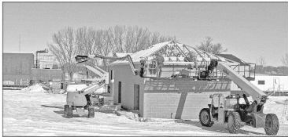
West Branch Construction of Boyden works on the roof for the Sheldon meter building for the Lewis & Clark Regional Water System. Work is slated to be done in October. Photos submitted
