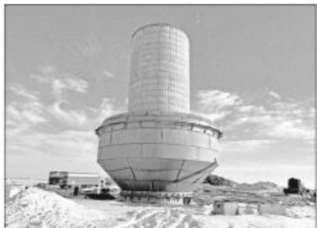
The welding is finished for the basin of the tower going up outside of Sheldon for the Lewis & Clark Regional Water System.
