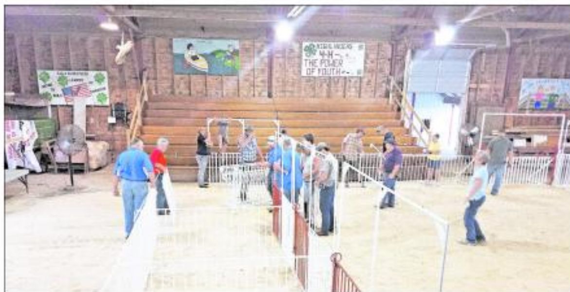
O'Brien County Fair Board members construct show pens prior to the start of the 2017 fair in Primghar. The board plans on upgrading the show ring with new lighting and a large ceiling fan to improve ventilation. Fair board president Darwin Gaudian and vice president Kevin Mars appeared before the board of supervisors on Tuesday, Jan. 24, to share details of the fiscal year 2023-24 budget and planned improvements to the show ring. Photo submitted
