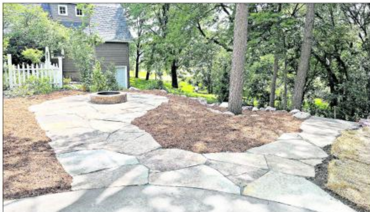
Hustedt Landscaping of Sutherland installs an outdoor firepit in Cherokee. Before installing, Business owner Brent Hustedt meets with clients to finalize landscaping designs and then prepares a digital, computer-aided preview.
