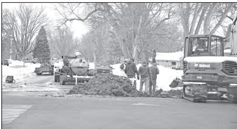
City crews examine a leak at Fourth Avenue Northeast and Seventh Street Northeast. It was one of three leaks the city repaired in the past week. Photo by Renee Wielenga
