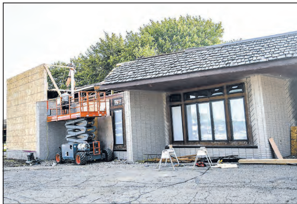
The north corner wall and roof of Sioux Center United Reformed Church has been rebuilt to make room for the Highway 75 redesign project. Along with that, the church is working to remodel the rest of the building's front. Photo by Eric Sandbulte
