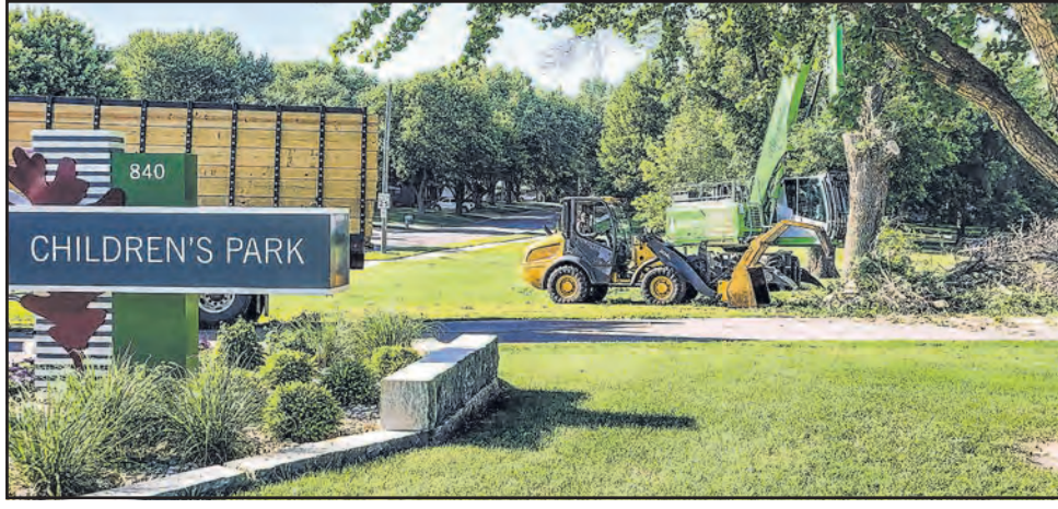
Heavy equipment works on removing ash trees from Children's Park in Sioux Center on June 19. The park had 35 trees taken down because they were too damaged by the emerald ash borer to save, temporarily closing the park. Photo by Eric Sandbulte
