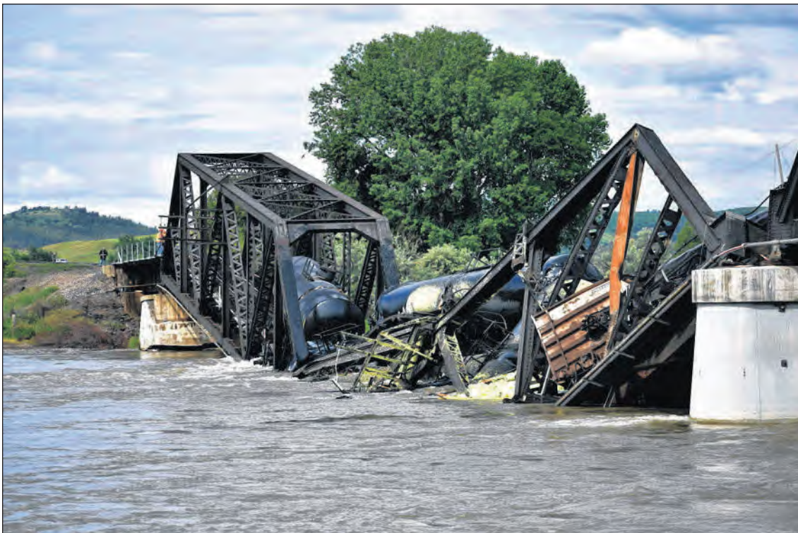
Several train cars are immersed in the Yellowstone River after a bridge collapse Saturday near Columbus, Mont. The bridge collapsed overnight, causing a train that was traveling over it to plunge into the water. (Associated Press)
