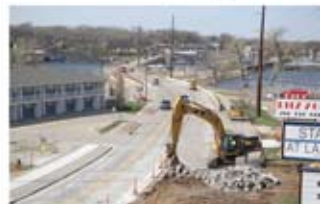
Contractors have removed concrete near a number of intersections in Okoboji and Anolds Park as part of a major project to repave about 2.5 miles of Highway 71. (Photo by Beth Boyce)
