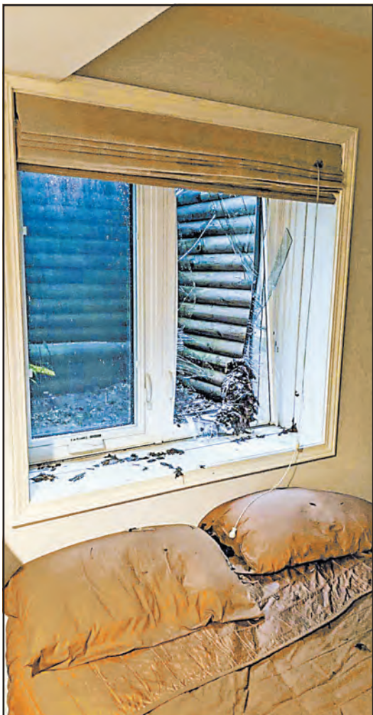
Floodwaters filled and broke this egress window, sending glass and debris into a basement room of Laura Heitritter's Sioux Center home.
