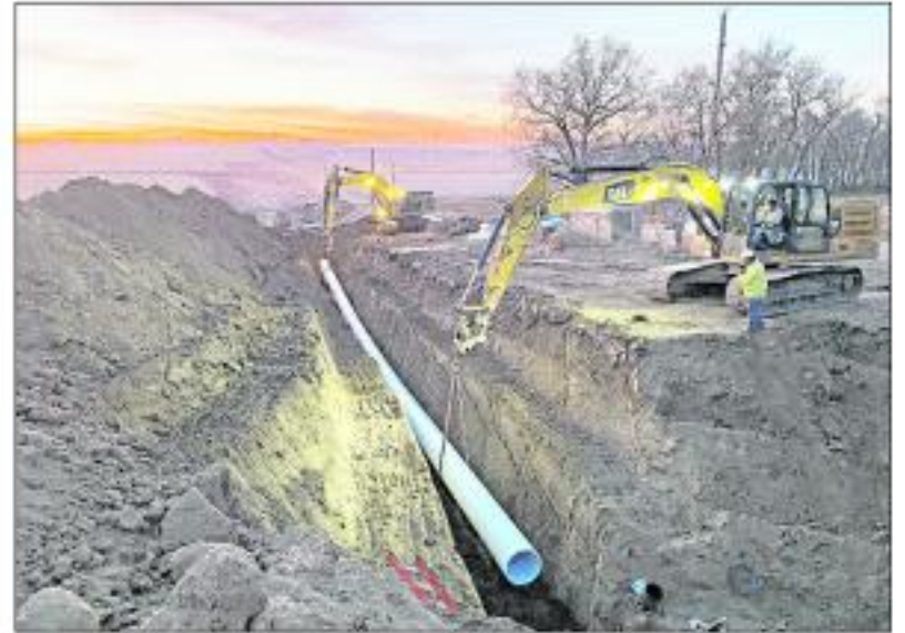
Excavators install PVC pipe between Beresford, SD, and Sioux Center in 2020. The pipeline has been completed, and water from the Lewis & Clark Rural Water System started flowing to Sioux Center on Tuesday. Photo submitted
