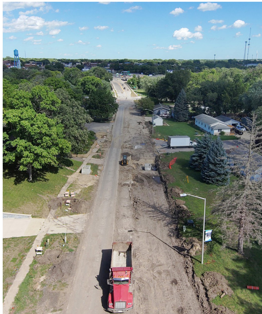
Road construction on Highway 9 continues to inconvenience Estherville residents and visitors, but with a little patience, it will all become a distant memory
