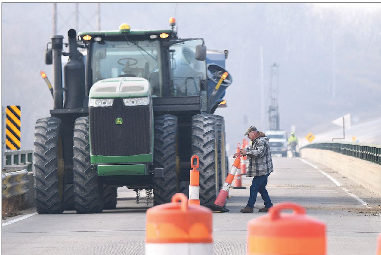
A farmer moves traffic cones Dec. 7 while trying to get a tractor and trailer across the Rochester bridge over the Cedar River. Allender Butzke Engineers closed one lane of traffic while conducting soil borings along the bridge in preparation for replacing the structure. The Cedar County Engineer's office stated that no wide loads — greater than 12 feet wide — would be allowed to cross during the work but engineers allowed the farmer through while traffic waited. Gregory R. Norfleet/West Branch Times
