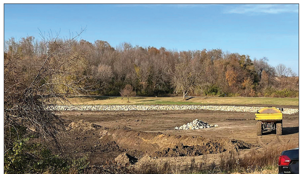
The southeast portion of Otter Creek Lake pictured in late October following the mobilization of Rachel Construction.
